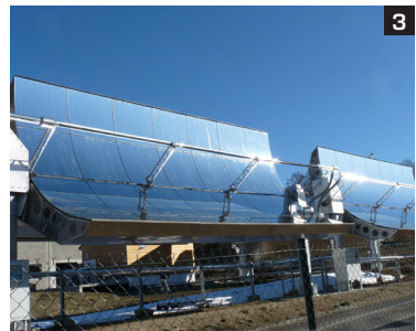
The 150 kW (thermal) small scale trough power plant
